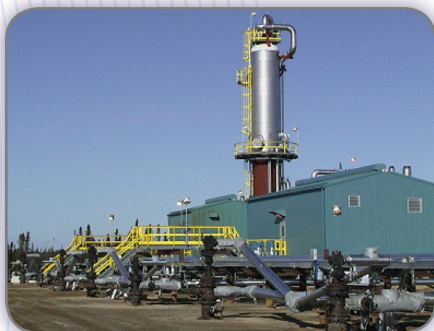
A typical SAGD wellhead, where steam is injected and a bitumen/water mix is extracted.
